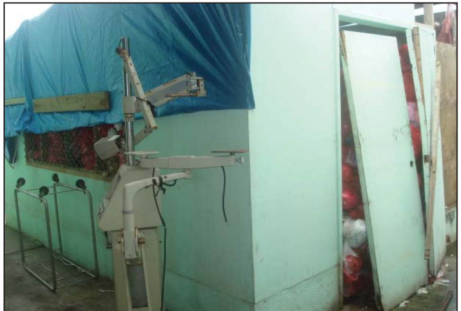
Bags of biohazardous waste peek out from behind the broken doors of the designated waste storage area.
