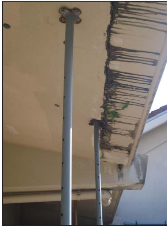
Metal supports have been attached to sections of the hospital’s exterior to keep the roof from collapsing.
