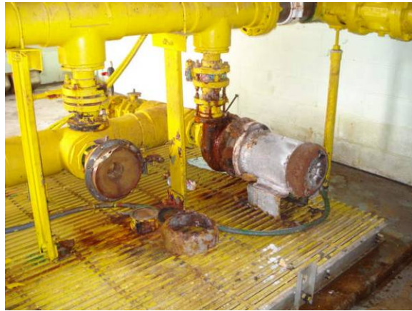
Lack of salt water pump
