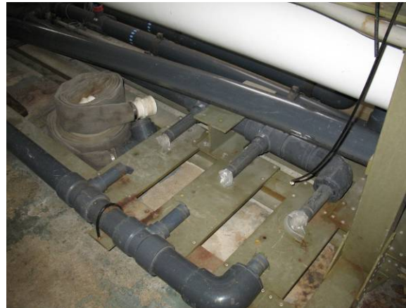
Needing replacement of parts
