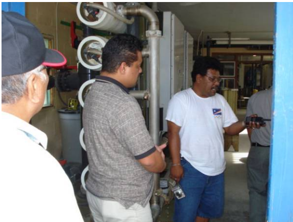
Reviewing the RO units
