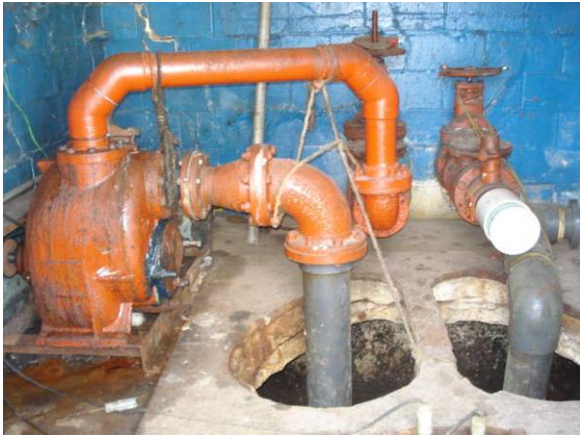
Old sewer pump
