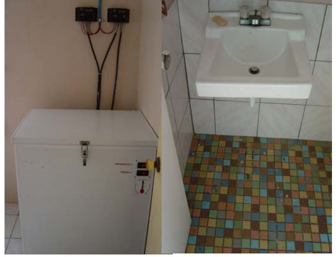
Solar powered Refrigerator & Sink
