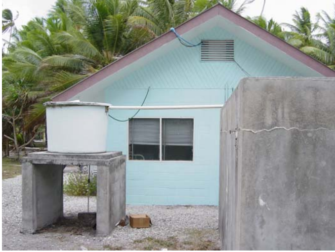
Health Center: Water tanks(Concrete & Fibreglass)
